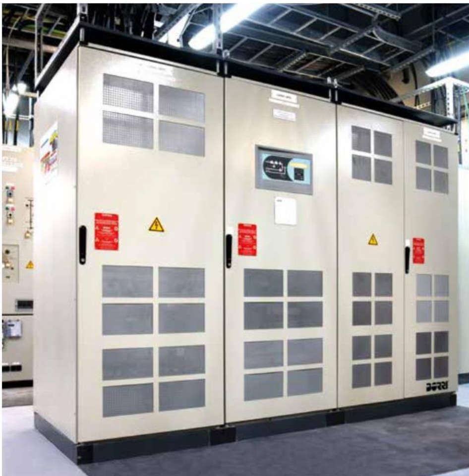
Borri AC UPS E3001.igbt 200 kW
